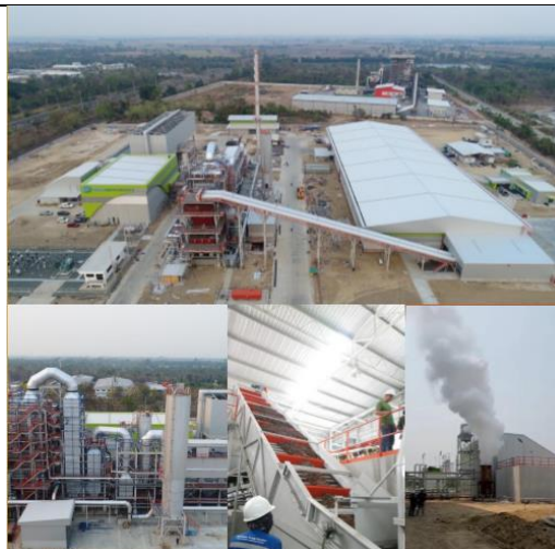
Figure 7: WTE projects in Thailand
